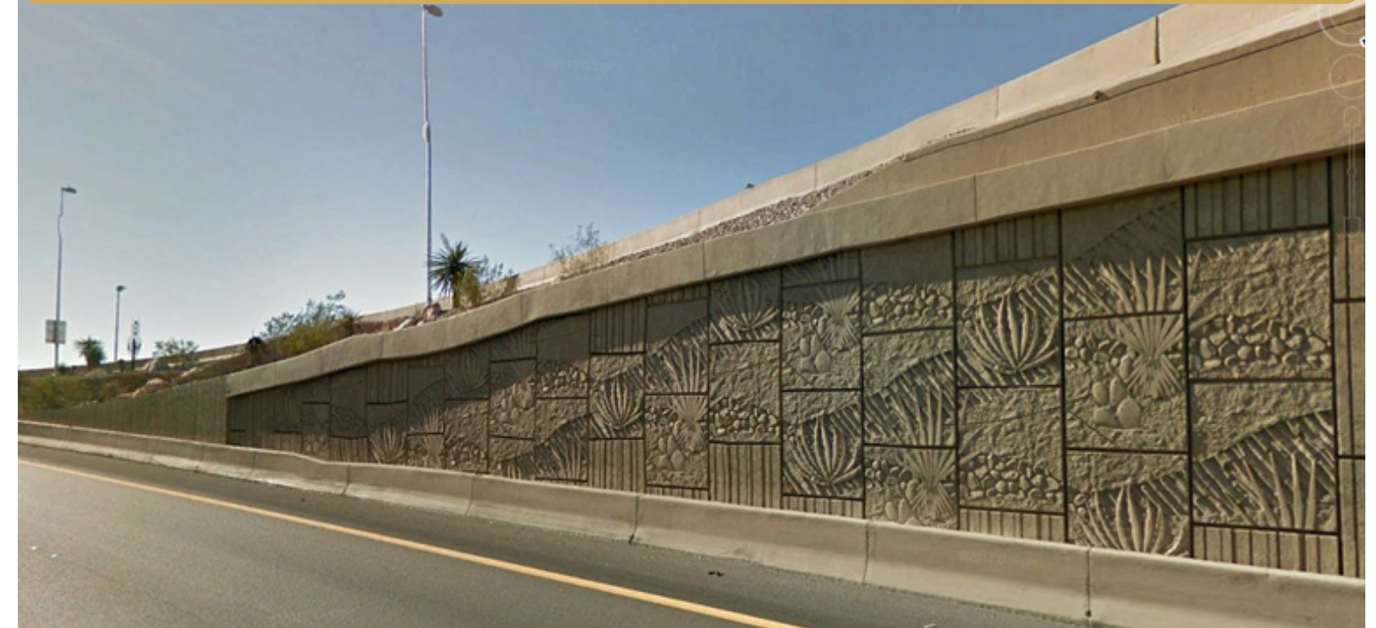
Figure 3.11 Example of color that would be used and type of decorative texture that could be used for retaining walls within the Henderson Interchange.
